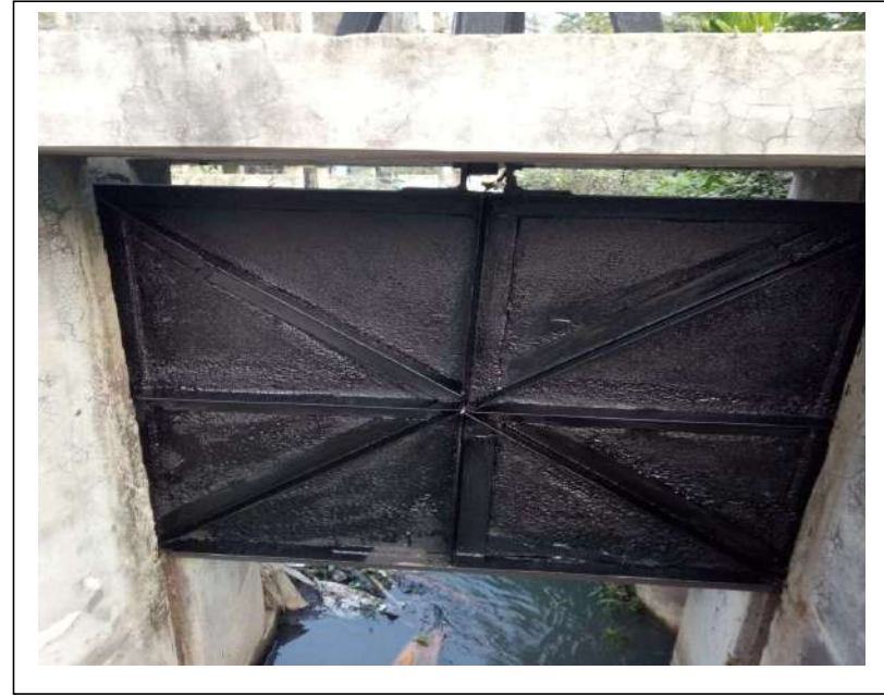
HALISAHAR DRAIN LOCKGATE
