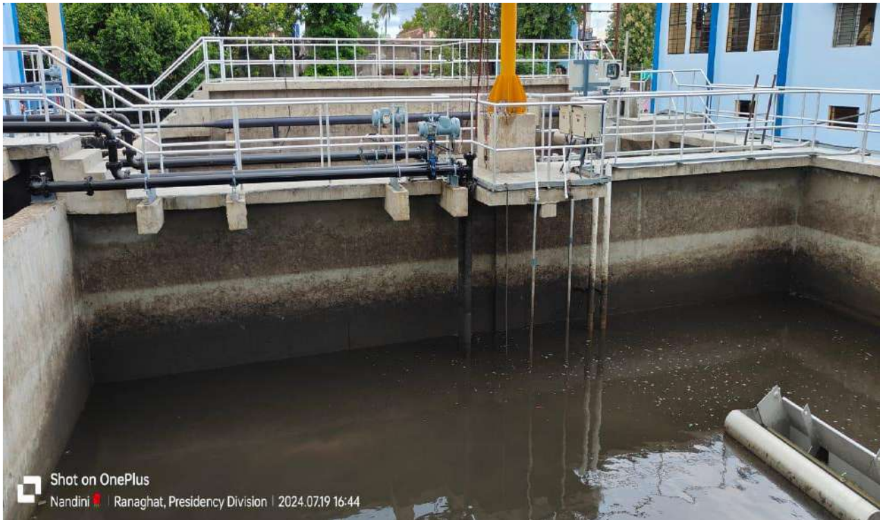
STP at Silver Jubilee Road - Ranaghat, Nadia
